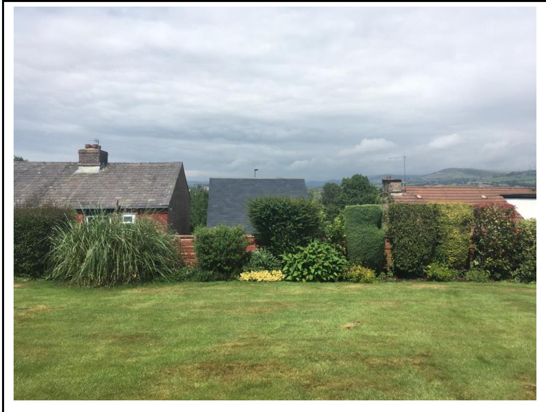
Roof, as seen from garden of neighbouring bungalow behind in Silver Springs
