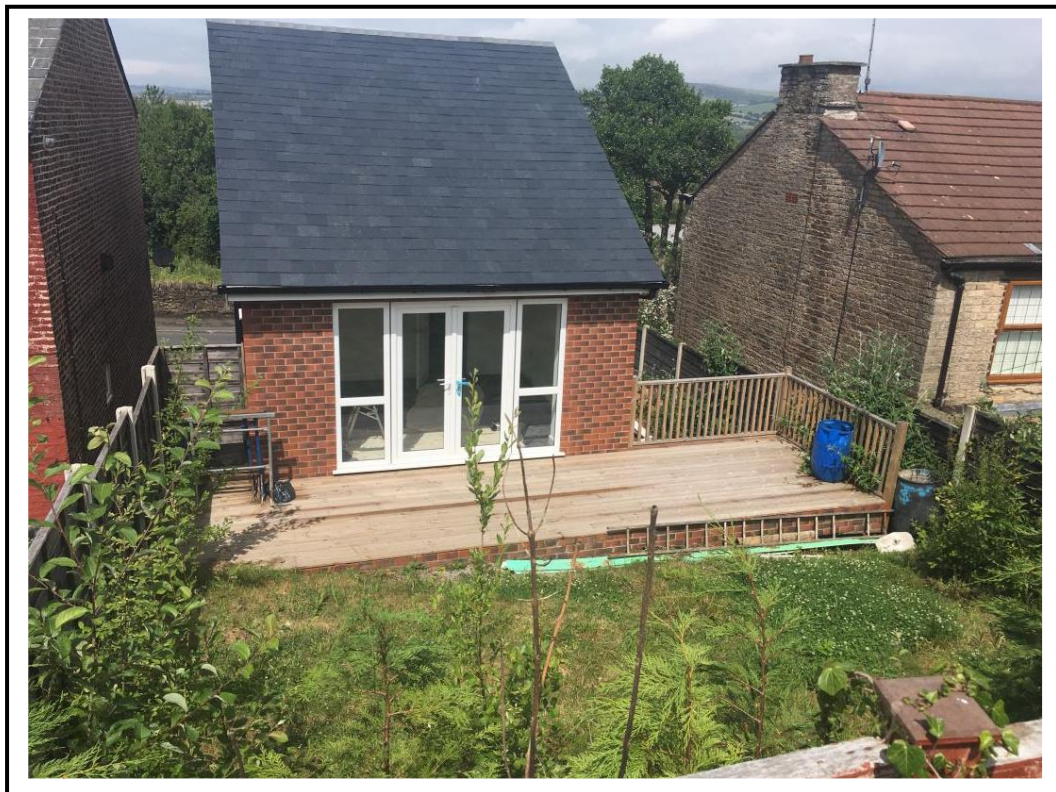
Rear elevation, facing towards garden of neighbouring bungalow behind in Silver Springs
